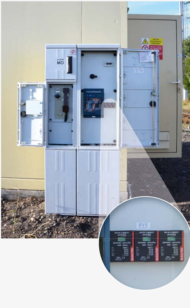
Fig. 2 Signalling system power supply pillar
